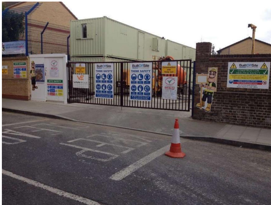
Figure 4: Example signage, to be displayed on the main entrance to the site
